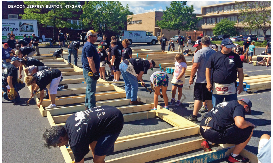
St. Mary's parishioners band together to help construct every wall used in Tabor House, a transitional home built in partnership with the Diocese of Gary and Habitat for Humanity. The home, located near the Cathedral of the Holy Angels in Gary, will provide a place for single-parent households to get back on their feet.
